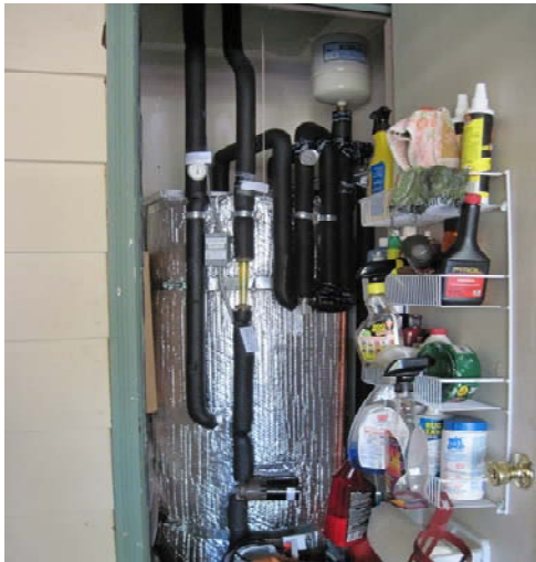
Solar Hot Water
