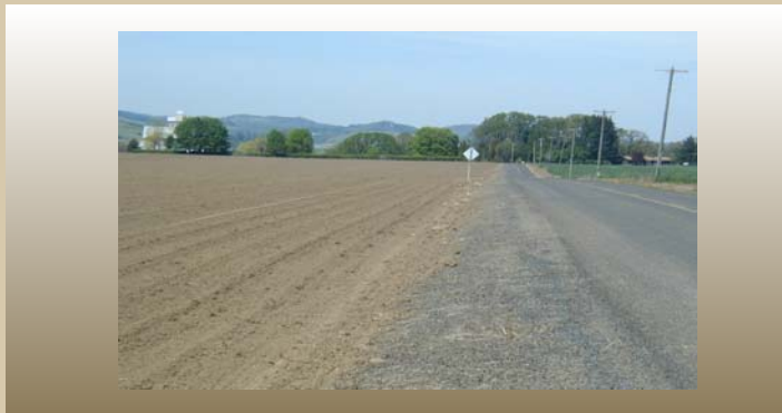
Lack of vegetation in ditch will lead to erosion.
