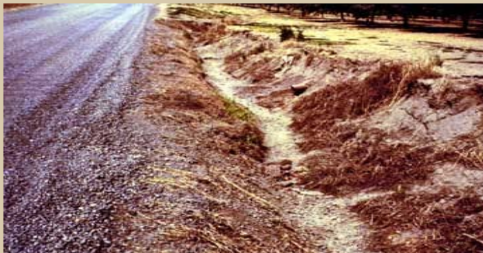
This eroding driveway ditch is obviously contributing to water pollution.
