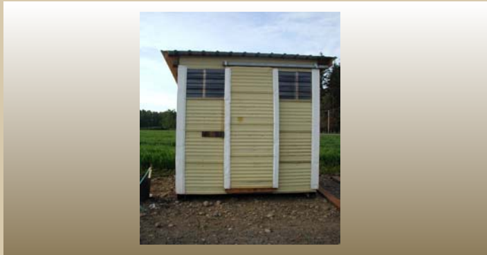
Chemicals are stored in separate building, but there are no warning signs.
